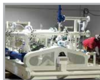
Closed Drain - Knock Out Drum liquor hydrocyclone feed pumps
