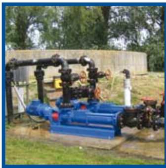
Transfer pumps at a WWTW's pumping sludge
