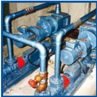
Packaged pumping system transferring raw sewage
